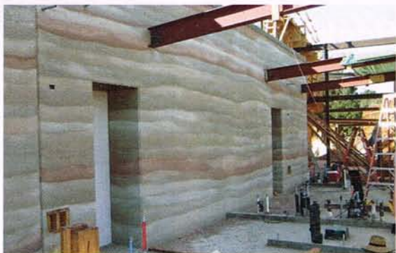
Mineral soils were trucked from several quarries to achieve the desired color coordination. Embedded steel columns support the adjoining floors and roofs.
